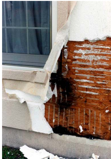
Figure 1. Rapid durability failure of wood-framed wall clad with barrier EIFS in the southeastern U.S. EIFS cladding is removed at lower right to reveal deterioration of wood-based oriented strand board (OSB) sheathing. The house is fewer than five years old at the time of the photo. Note the localized deterioration of the wood-based sheathing (black areas) beneath locations of leakage at window-frame corners and window-perimeter sealant joints.
