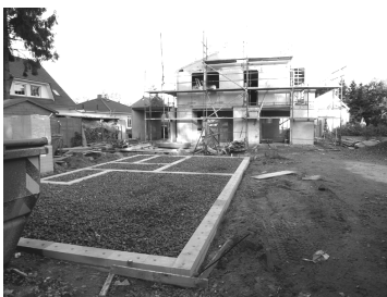
Figure 9. Behind: Building carcass of the main house. Front: Foundation of the subsidiary house.
