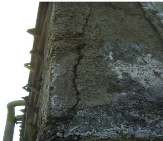
Figure 3. Longitudinal cracking and sulfate attack
