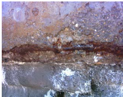
Figure 4. Severe corrosion of reinforcement
