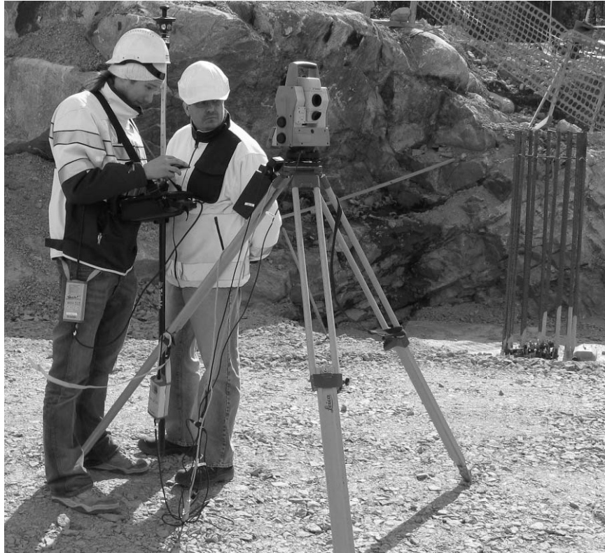
Figure 5. The prototype system at the field test site. Measured bridge foundations in the background (right).
