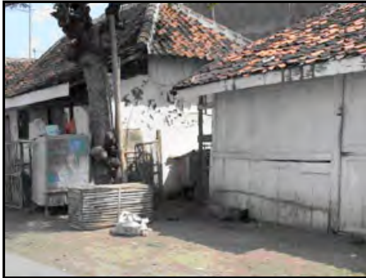
Figure 5 The damage of wall in vernacular house of fisherman in Sidopekso Kraksaan Probolinggo
