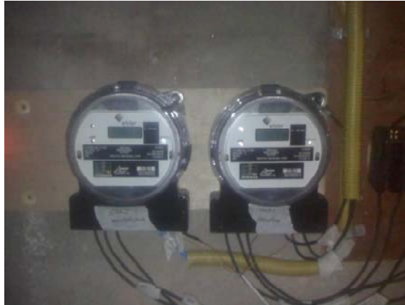
Figure 2 - Electrical energy meters used
