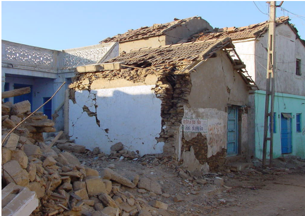
Figure 4 catastrophic Failure of Wall Constructed with Bricks and Mud Mortar in 26 th January 2001, Bhuj Earthquake.
