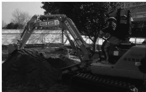
Figure 11 shows a humanoid robot riding an excavator
