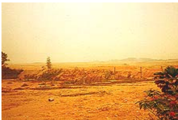
Figure 3: Land clearings for building construction especially for terrace houses due to uncontrolled urban development near Kuala Lumpur.
