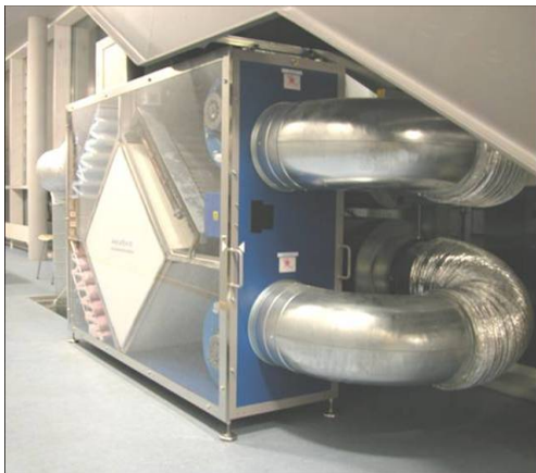
Figure 3. Air Handling Unit (AHU).
