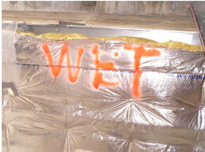
Figure 6. Water-damaged duct riser – marked for removal.
