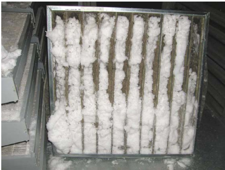
Picture 1. The filter blocked up with snow.
