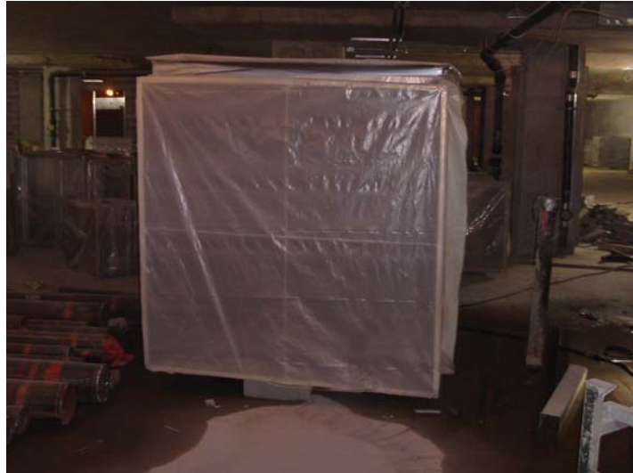
Figure 3. Proper AHU storage – pre-installation.
