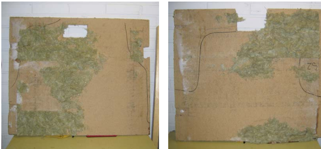
Figure 5 Condensation and frost with mineral wool pieces on the inner surface of the sheathing of the attic floor on the timber-frame wall (left) and the AAC wall (right) cases.
