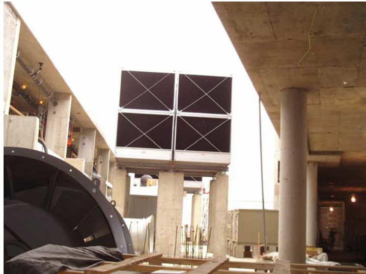
Figure 5. Cooling tower installation.
