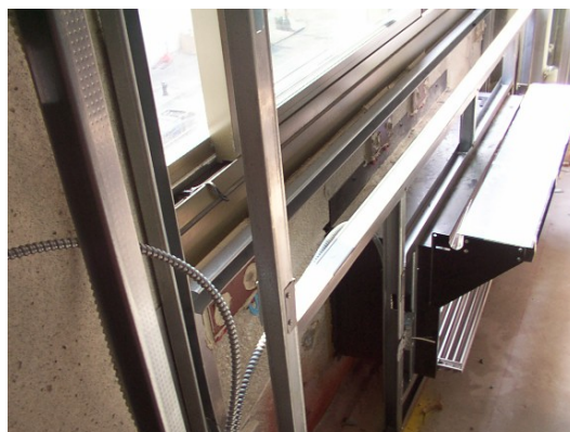
Figure 1. PTAC unit housing in multi-story residential building.
