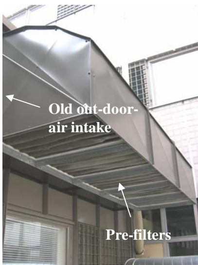
Picture 4. The pre-filter used for prevention of the snow entrance.
