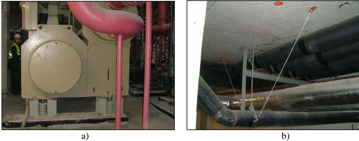
Figure 6. Applications of seismic isolators (a) and seismic cables (b) in Canyon Levent
