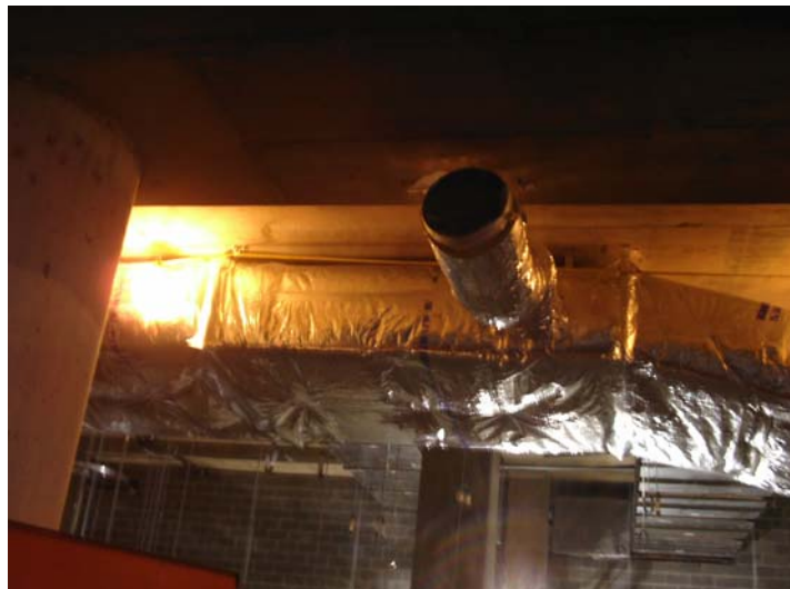
Figure 4. Protected branch entry duct opening.
