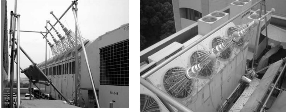
Figure 3. Thermal flux samplers mounted on VRV system.
