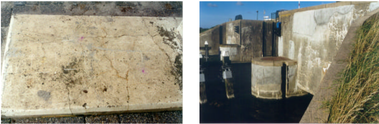
Figure 1: ASR-attack in the foundation of a viaduct (left) and a lock (right) in the Netherlands.
