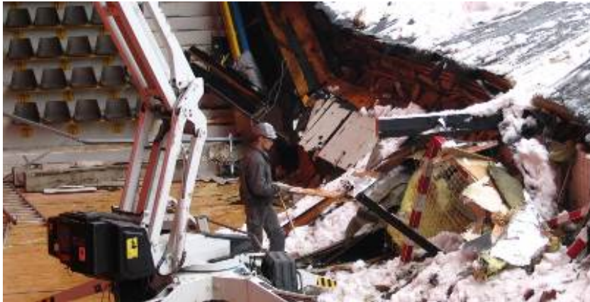
Figure 3: Damage to a sports arena after the roof collapsed, caused by heavy snow loads in 2007
