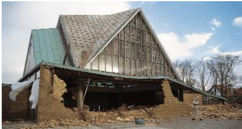
Figure 2: Damage to a building after the heavy windstorm passed over the southern half of Denmark on 3 December 1999
