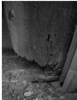
Photo 9. Decayed Column Base
