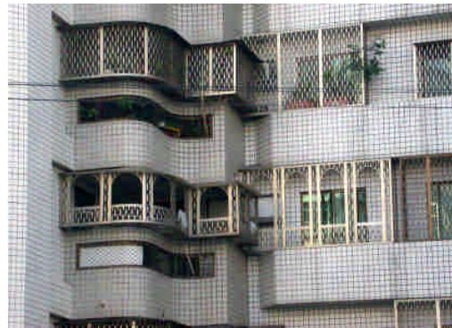
Fig. 7 Railing not for Protection
