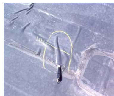
Figure 2. Ripples in an EPDM Membrane and Seam
