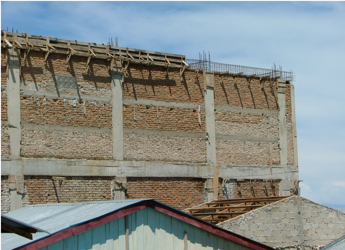
Figure 7. The above 2 level building in Nias has a deep ring-beam at the top of the wall, numerous stirrups and reinforcing rods, beams and columns with wide dimensions, and two intermediate beams in the brick panel walls. It is located on soft ground and also has excellent foundation ground beams. Observations of similar undamaged buildings indicate it should survive very strong MM9 to 10 intensity shaking without collapse.
