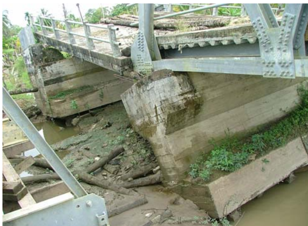
Figure 5. A bridge pier and abutment damaged by liquefaction and lateral spreading causing settlement and rotation. The bridge superstructure is well designed and undamaged but unfortunately can no longer be used because of the abutment and pier deformation.
