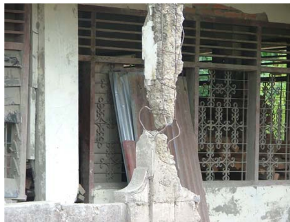
Figure 6. Structural failure due to light reinforcing and wide spaced (lack of) stirrups - a common problem
