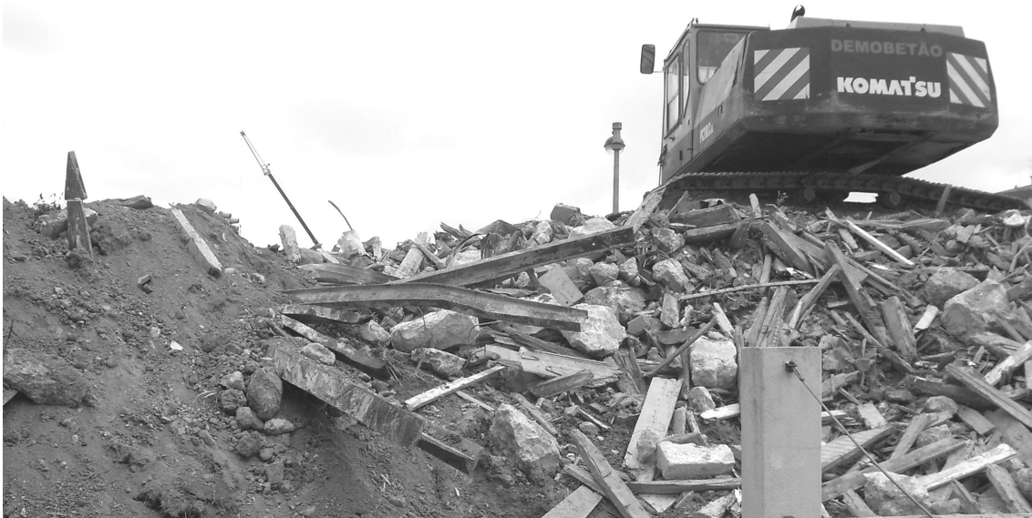
Figure 2. Typical early XX century building under demolition in Lisbon. Notice large percentage of soil content, with mixed metal, stone and wood elements
