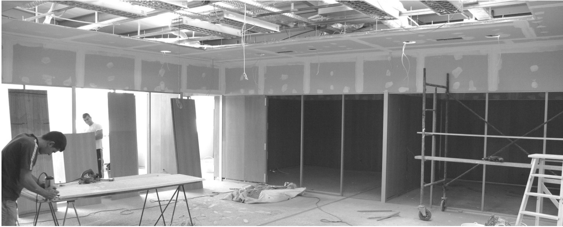
Figure 4. Work in progress at the new IP offices in Cacém (March 2006). Doors, wood veneer wall panels and all lighting fixtures were being reused after disassembly from original location in Lisbon.
