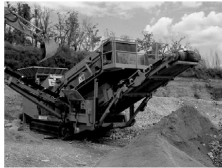
Figure 3. Mobile plant composed by a single machine with crusher, magnetic separator and vibrating screen
