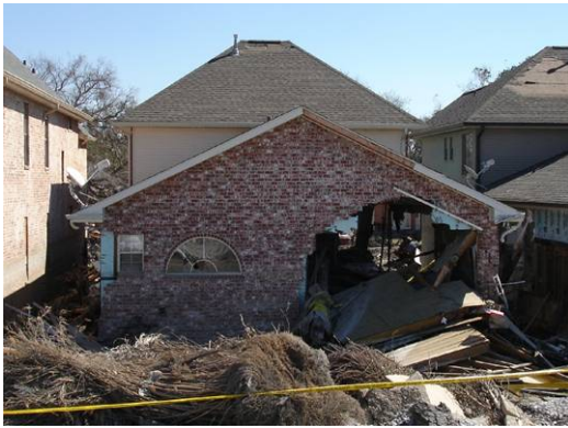
Figure 4. Brick clad wall damaged in vicinity of a levee breach.
