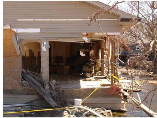
Figure 5. Wall clad with vinyl siding damaged in vicinity of a levee breach.
