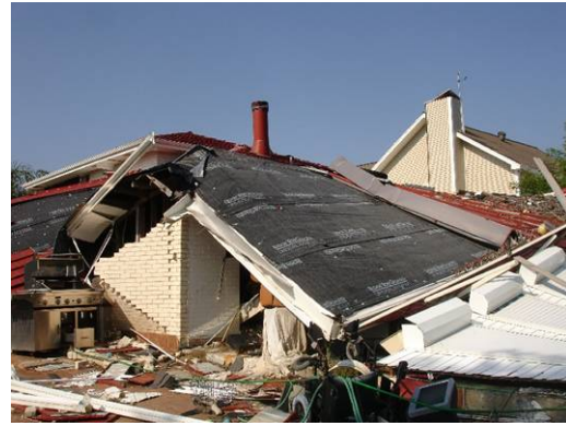
Figure 8. Porch collapsed from uplift forces and lack of tie downs.
