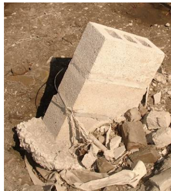
Figure 2. Foundation pier without evidence of mechanical connection.
