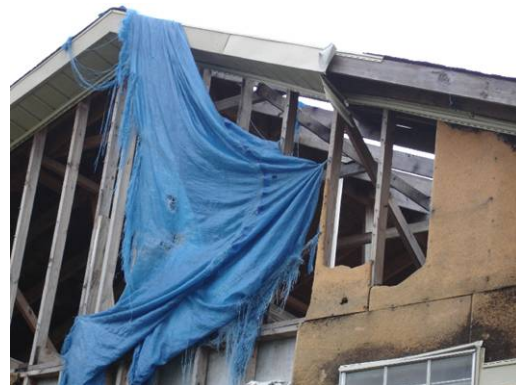
Figure 10. Poorly fastened sheathing that was blown off of a gabled end wall.
