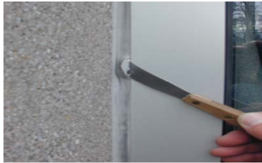
Figure 3. This is an example of the type of “invisible” seal failure uncovered by using the non-destructive method and device described elsewhere in the paper. Prior to finding this seal breach, the entire sealant bead depicted looked exactly like the area above and below the breach.
