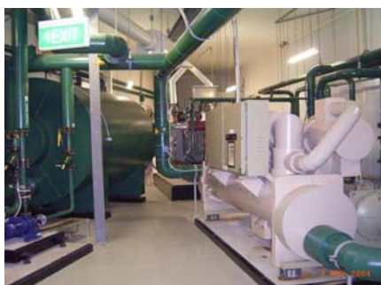
Figure 3. The Plant Room
