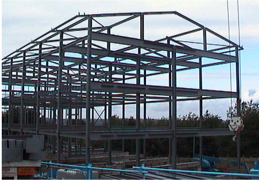
Figure 8a. 'Actual' Progress of work on the School of Health Project at Week 15 of mobilisation to site
