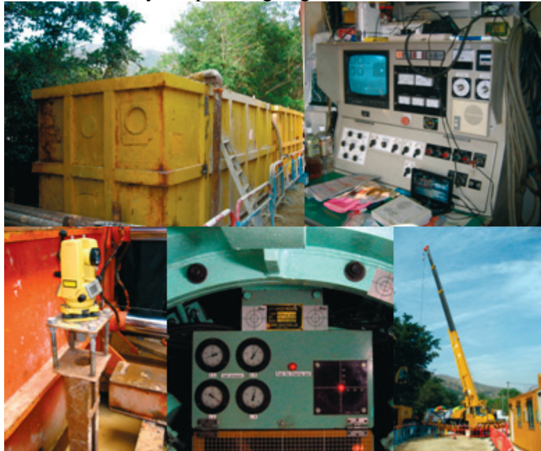
Fig. 6 – Sedimentation tanks (top left), operations system (top right), total station (bottom left), target board (bottom middle), Crane (bottom right)
