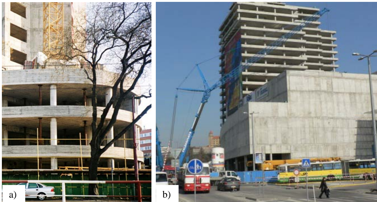
Figure 4: a) Crane on Ceiling Structure of the 3th floor – Gloria Bratislava, b) Removal of Crane Tower from Structure – Aupark Bratislava
