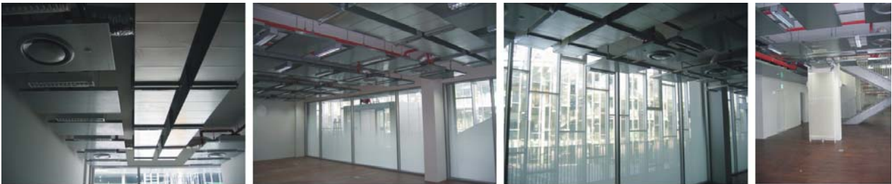
Figure 9 Indoor spaces of CCA system and cooling radiator
