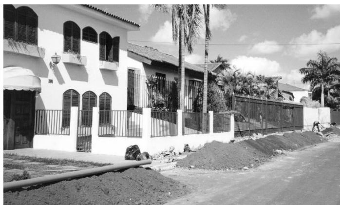
Figure 1: Simplified sewerage being installed at the back of the pavement in Brasilia
