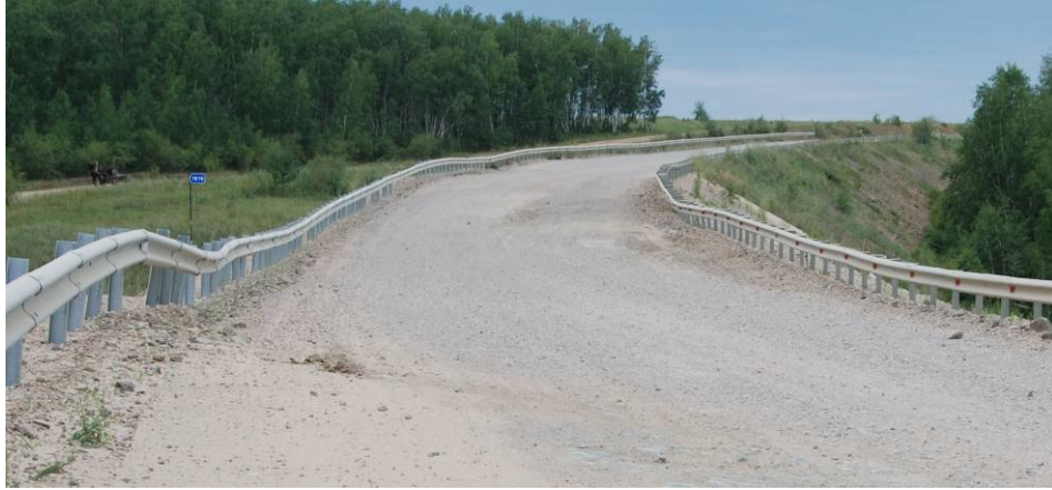
Figure 2. Section of highway "Amur", km 247, 23 months after innovation repair, August 2008
