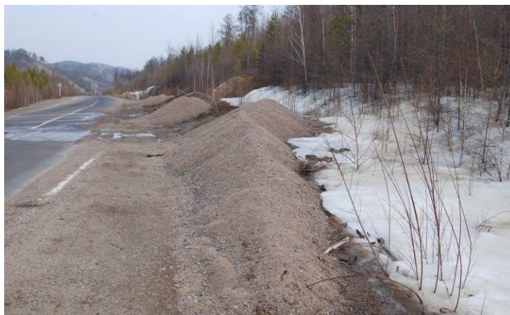
Figure 3. Icing on highway "Amur", km 89, April 2009
