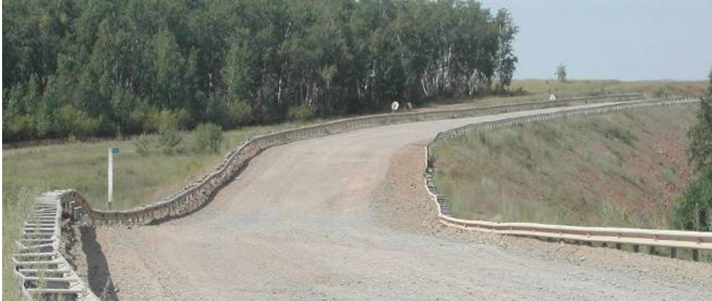
Figure 1. Chita-Khabarovsk highway deformation, 247 km, due to degradation of icy permafrost soils in the base, before the innovation repair, July 2006
