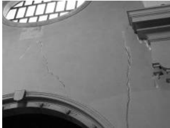
Figure 5: Vertical cracks in the interior face of the central nave wall
