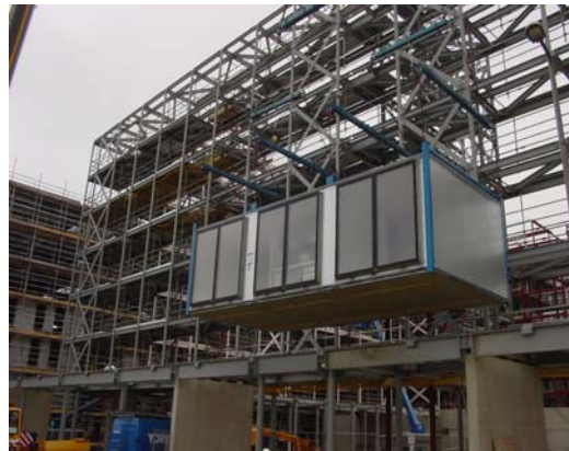
Figure 2: Open sided module with corner and intermediate posts supported by a structural frame (courtesy Yorkon and Joule Engineers)
