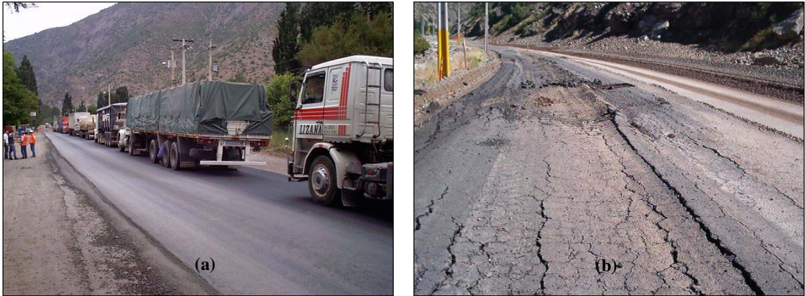
Figure 5: Rubblized section (a) end overlay section (b) after the rain
