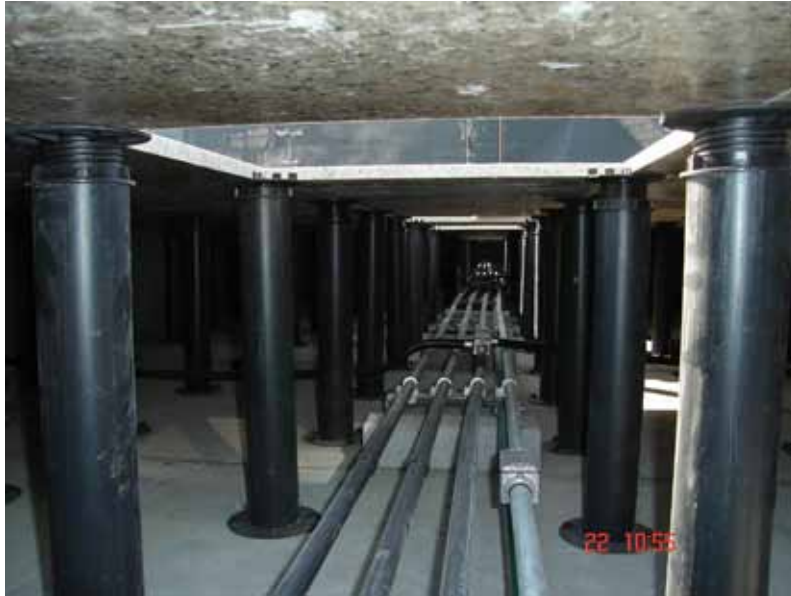
Fig.4 – Installation embedded in the drainage void area of a pedestal system in a commercial building in the City of São Paulo (Bernardes 2009).
