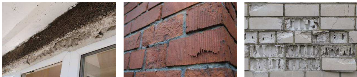
Figure 1. Frost damages of concrete (left), ceramic (centre) and calcium silicate brick (right) facades.
