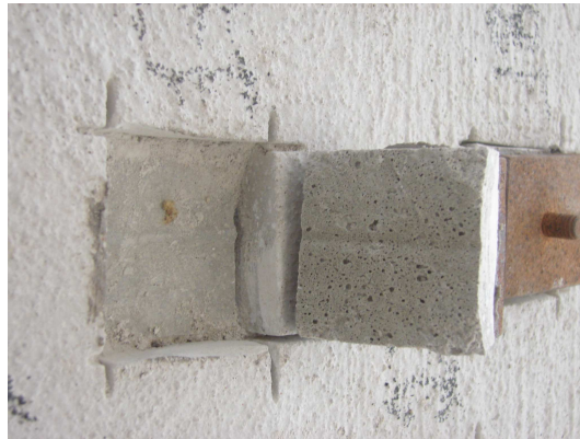
Figure 8. Condition of the main rupture occurring on the interface between the roughcast and the concrete substrate.
