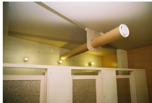
Figure 2: Card tube used for air supply in toilet
