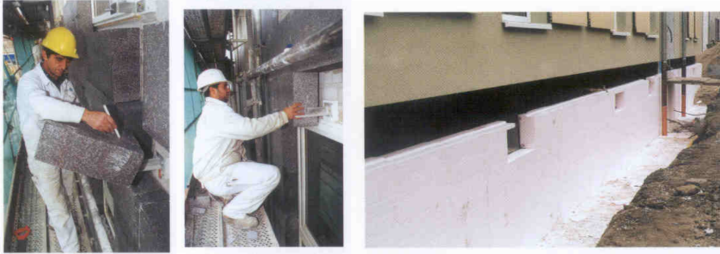
7., 8.,9.: The entire shell of the 3-Liter House is encased in thermal insulation.
