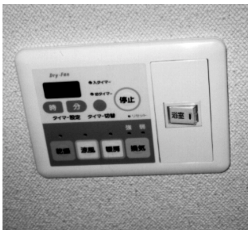
Photo 13. Bathroom controller is clearly visible.
