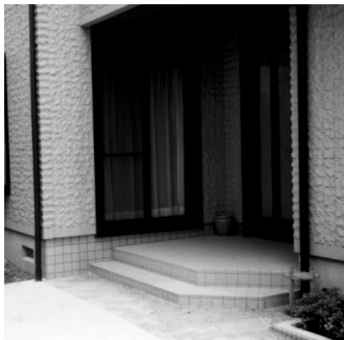
Photo 1. Entrance to the house. A handrail was installed afterwards to negotiate steps.
