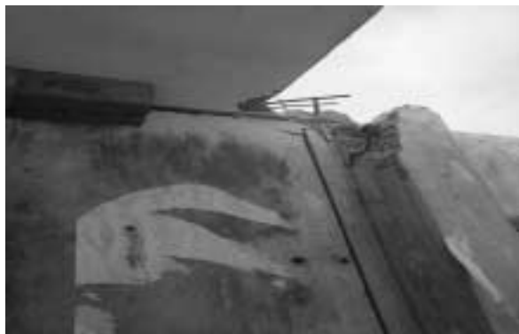
Fig. 11: The newly settlement of the construction after sawing the wall in two sections. The right section will be removed.
