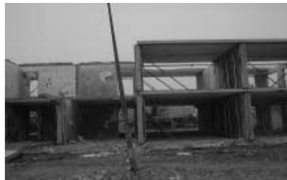
Fig. 12: After removing the floor it is clearly to see that the wall is not standing 90°. This will be fixed during construction
