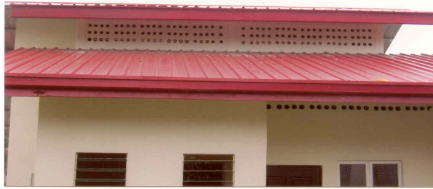
Figure 2 Ventilation gaps in the OPS house.
