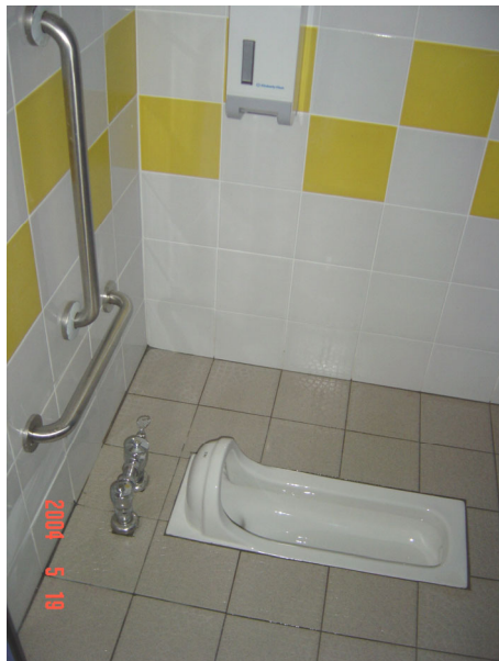
Photo 3 - The inverted T-shaped handles and an extension squatting toilet
