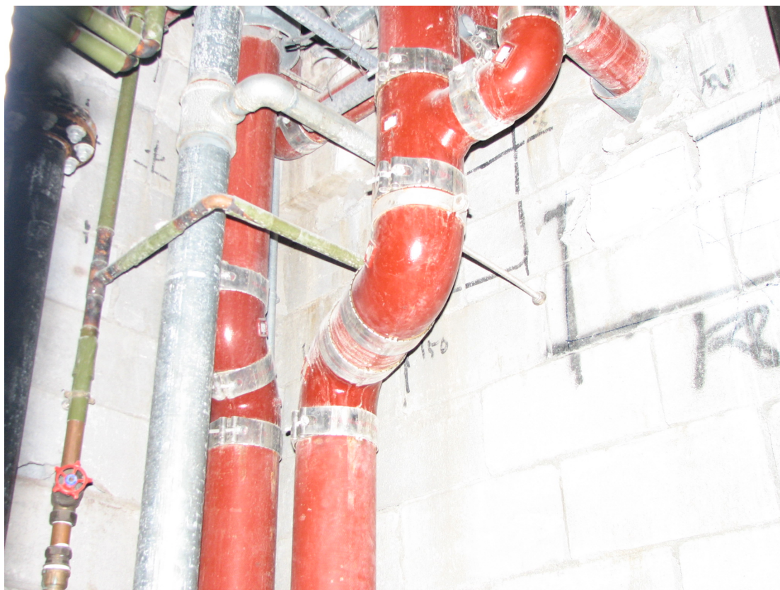
Figure 2 Unnecessary bendings along the vertical drainage stack
