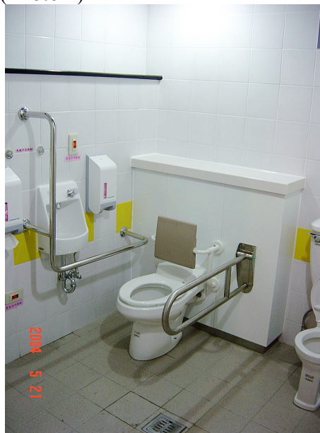
Photo 1 - The disabled toilet with a backrest without water tank. A small washbasin next to it, the width of two handles is 70 cm and height of 65 cm. (228 Park in Taipei)
