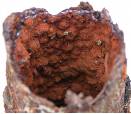
Figure 2 – Uniform corrosion of galvanized pipe
