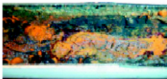
Figure 2. Discrete deposits on interior of steel pipe. These deposits are formed by microbes depositing materials from water and by the accumulation of corrosion products.
