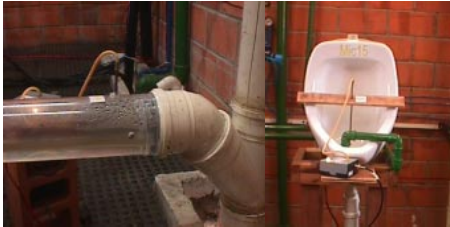
Vertical stack entrance
