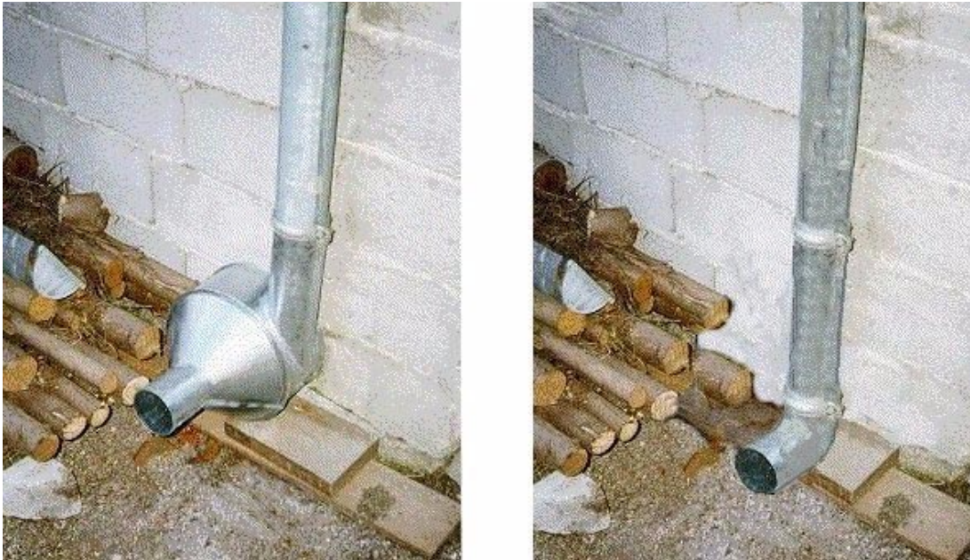
Figure 7. Water outflow instalation in house
