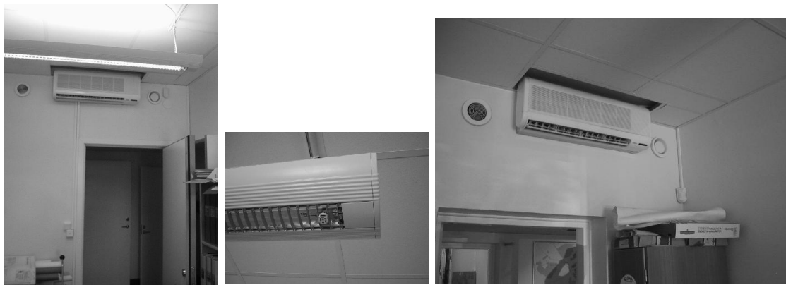
Figure 2: The test room installations. For the end-users' convenience the control of the heating fan coils and the lighting and their different combinations are in focus in the design and testing of forgiving technology.
