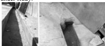
Figure 9 - The interior channel and the drain discharging water from concrete clad flat roof, B2.
