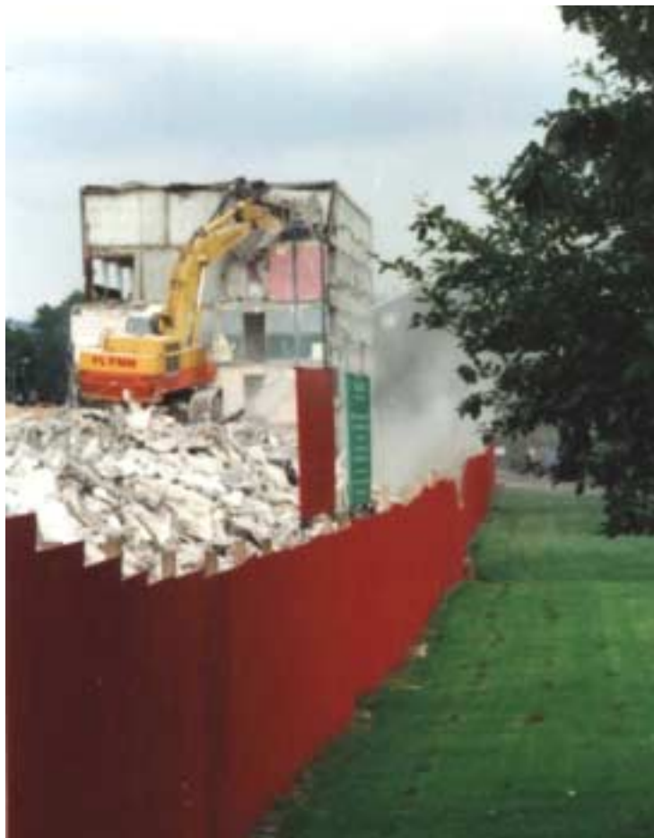
Photo 3. The 75 tonne excavator gains the height it needs using the debris pile.
