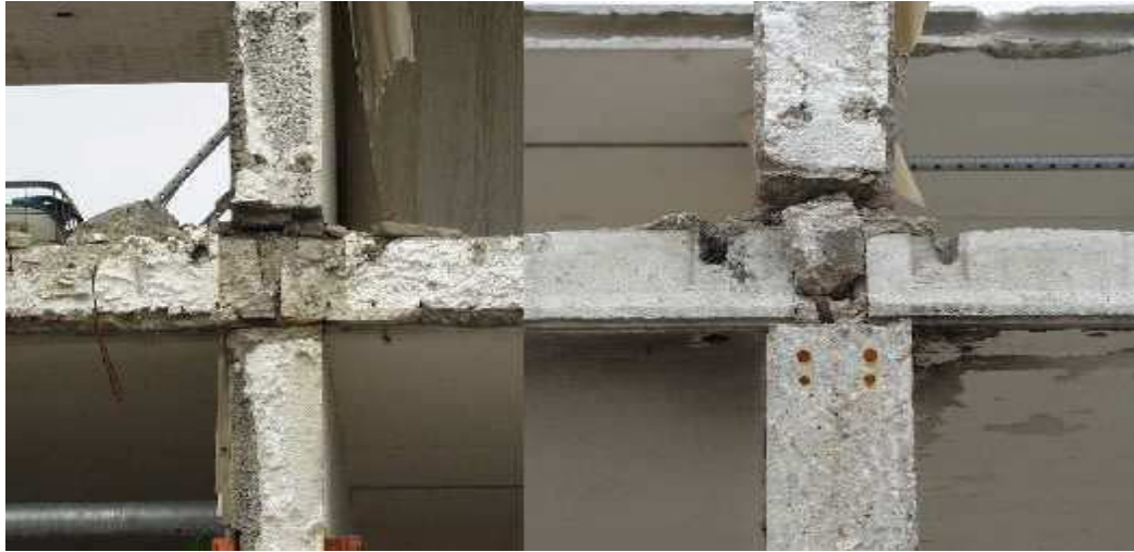
Figure 6: On the left the correct detail, on the right the detail which gave problems during the dismantling.
