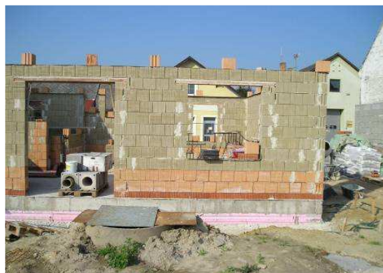
Fig. 4 Fired window and door lintel with 25 cm bearing support at each side
