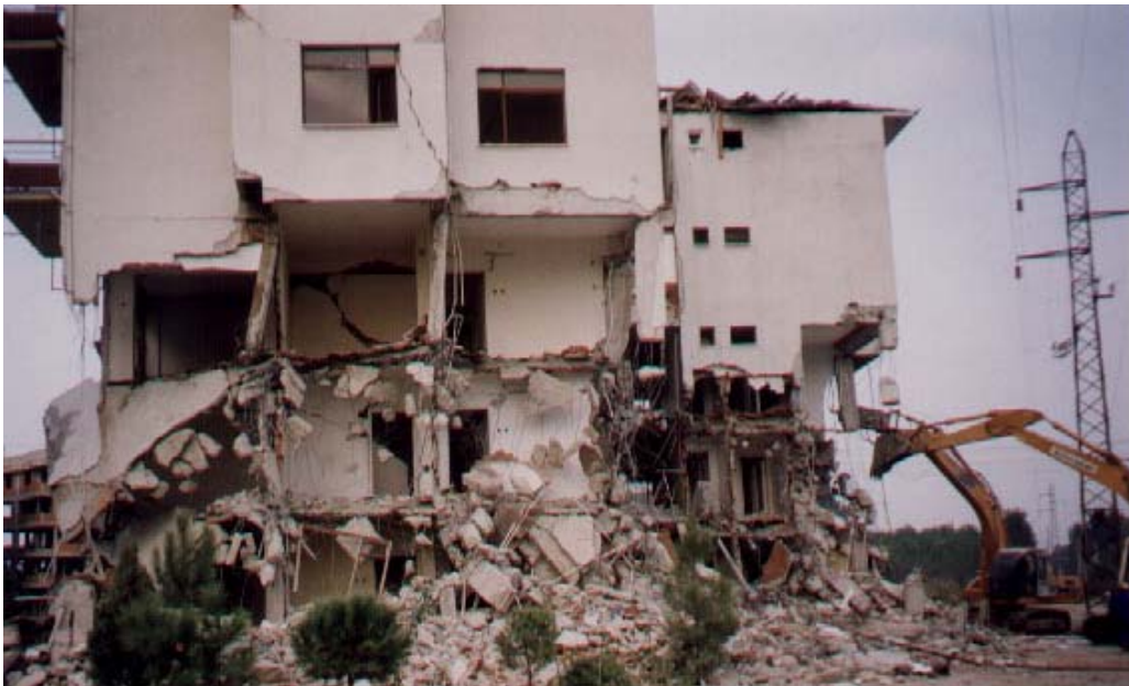
Figure 8: Columns of a building being pulled out in Gölcük [iv].
