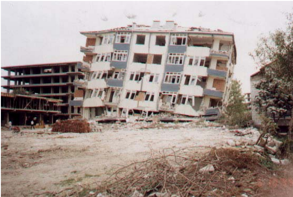
Figure 12: Building material being recovered from a dangerously damaged building: roof tiles stacked in the foreground (Gölcük) [i].
