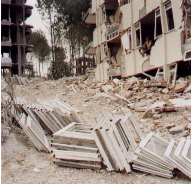
Figure 13: Rear view of the building in Figure 12 shows men working in this dangerously tilted structure to dismantle building components and fixtures; salvaged fenestration units are seen collected in the foreground [i].
