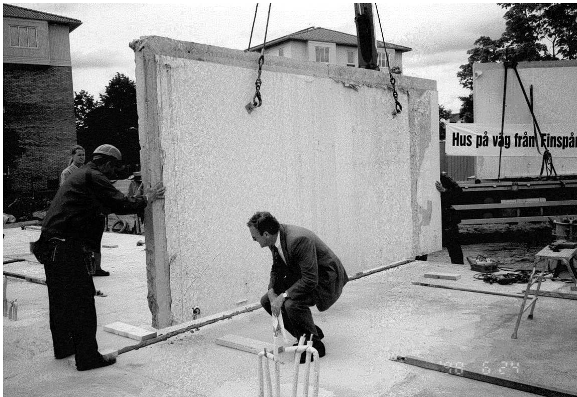
Figure 2. Concrete elements cut from cast in-place concrete walls delivered to the building site in Linköping under the supervision of the county governor, Björn Eriksson.
