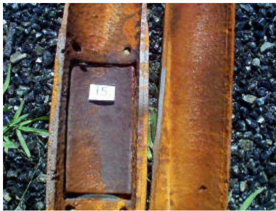
Figure 8. Close up of sample 15 from building 16 showing inspection cover and small through-wall defect on bottom right hand photograph.
