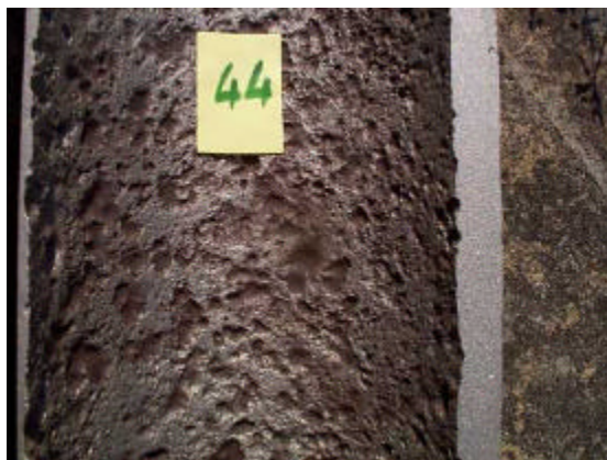
Figure 9. Close up of sample 44 from building 11 showing pitting corrosion. Also note the eccentric wall thickness.
