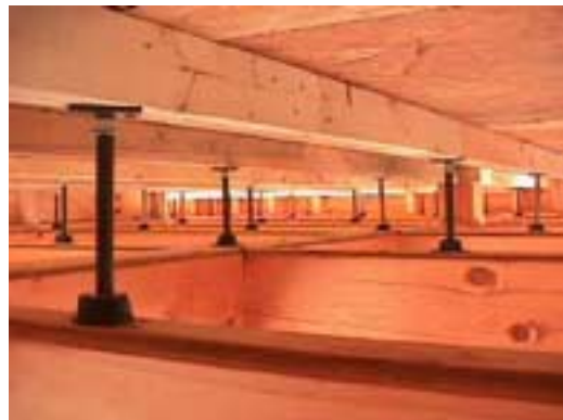
Figure 4 – Access floor seen from below
