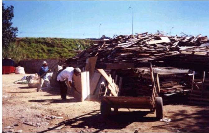
Figure 2 Wood being sorted at a CDW transfer station in São Paulo. Source: Pinto, T.P.
