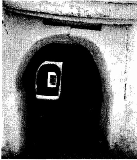
Figure 6: Pedestrian street with light shafts and cracks
